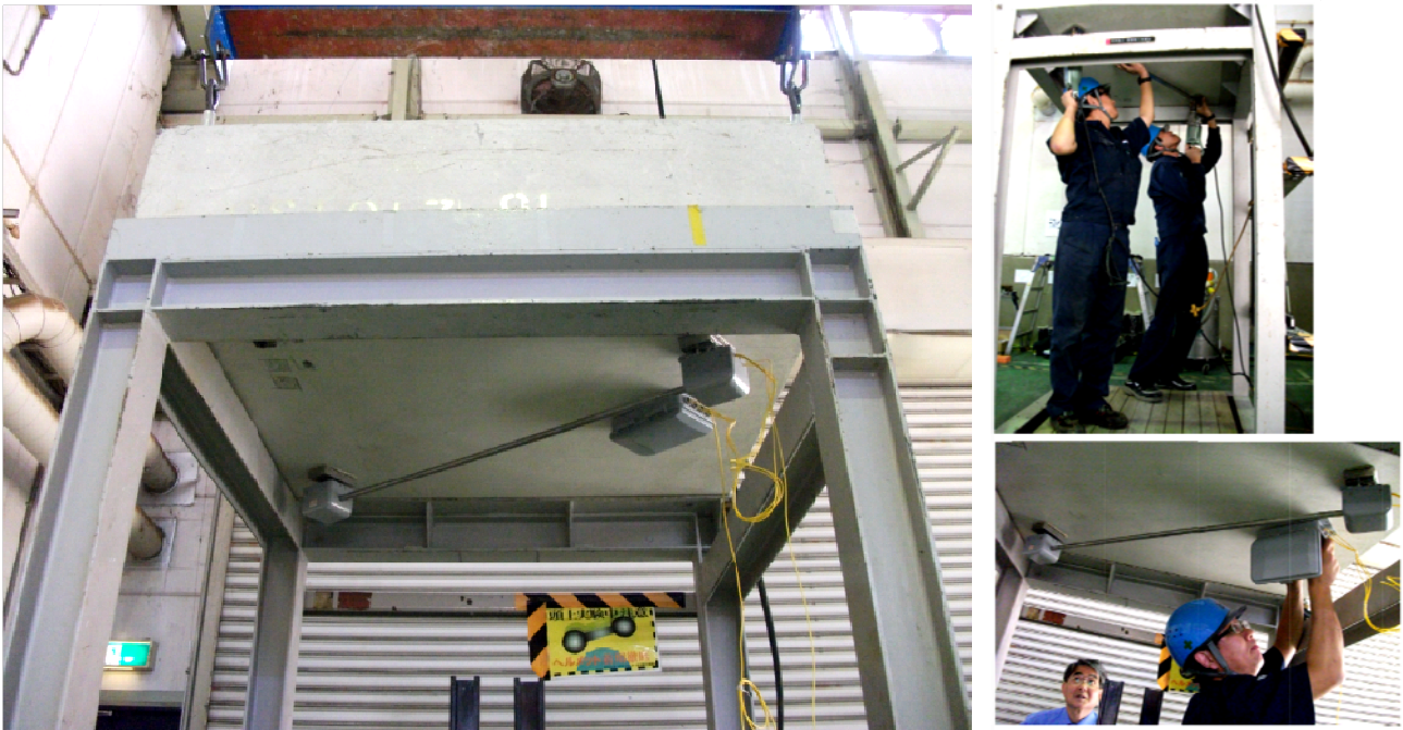
Pic-4 Setting the long gage sensor main unit and terminal box onto the concrete block object
