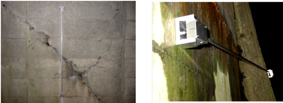
Pic-8 Situations of cracks and of the degradation of the tunnel And setting of the long gage sensor (old version) onto the concrete wall of the tunnel
