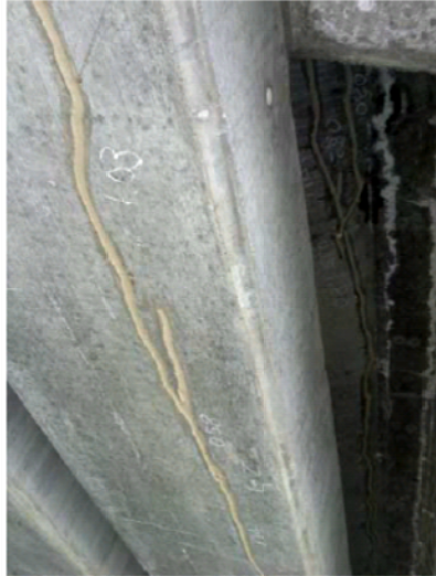
Pic-7 Cracks via the alkali-aggregate reaction
