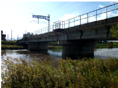
Pic-5 Decrepit Prestressed Concrete (PC) Bridge
